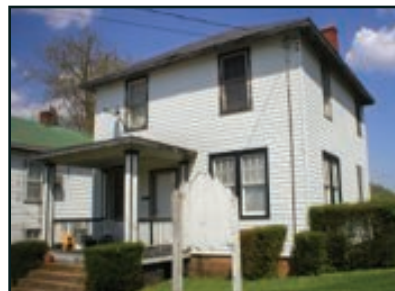
189 Main Street Issues: maintenance (railing, roof) Action: Minor Renovation - Complete
