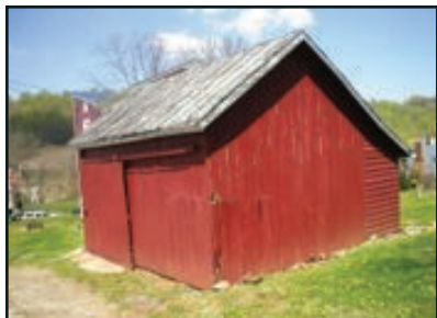
658 Front Street Issues: maintenance (rot) Action: Minor Renovation - Complete
